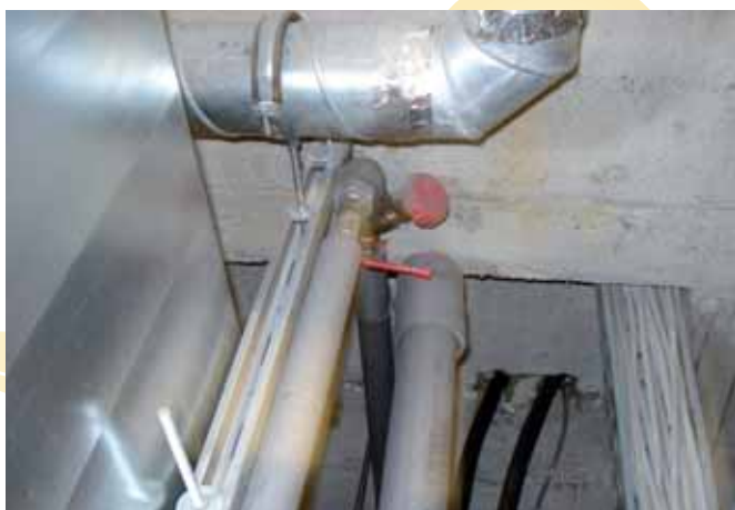
Hidden closed loop in hot water circulation system that provided room for Legionella growth — Source: OMF1
